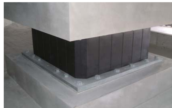
▲Multilayer rubber bearings incorporated into the seismic isolation system
